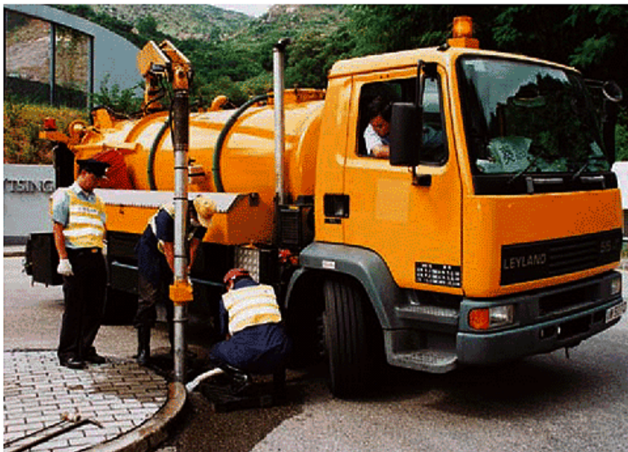
機動清渠車清理公路兩旁和繁忙街道的溝渠。 Mechanical gully emptiers are deployed to clear gullies along highways and busy streets.
