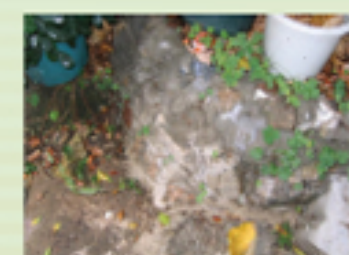
Fig.6.22 Cracks and crevices between rocks paved
