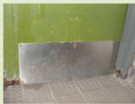
Fig. 6.14 (Right) Lowering of threshold clearance by installation of kicking plate on door.
