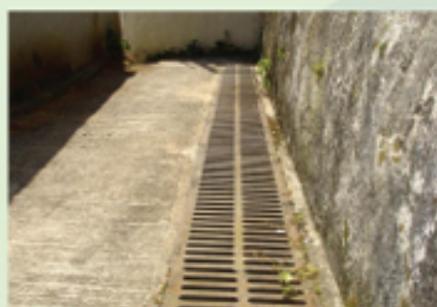
Fig. 6.9 (Left) Gnawed runway used by rodents inside surface channel.
