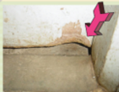
Fig. 6.7 (Left) Gnawed wooden door used by rodents as entry point
