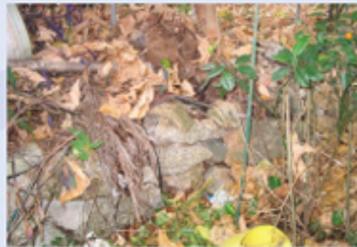
Fig 5.7 Cracks and crevices found between rocks of planter
