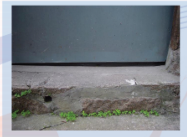
Fig 5.2 Threshold clearance of door larger than 6mm allowing rodent passage.
