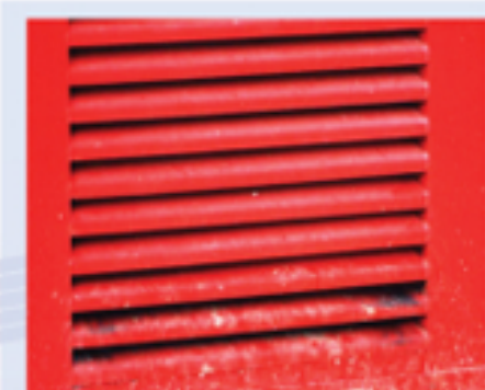
Fig 5.4 Ventilation louvers provide entry points for rodents.
