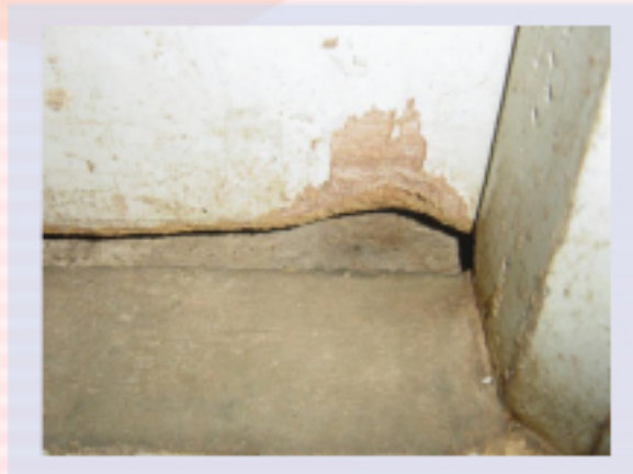
Fig 5.3 Damaged wooden door
