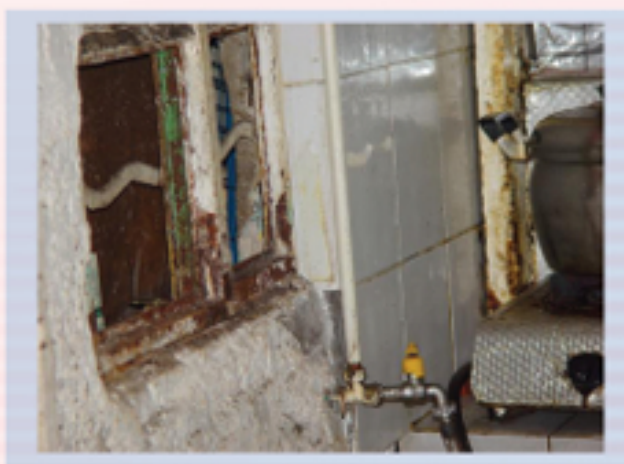
Fig 5.1 Broken windows provided rodents with passage to infest houses.
