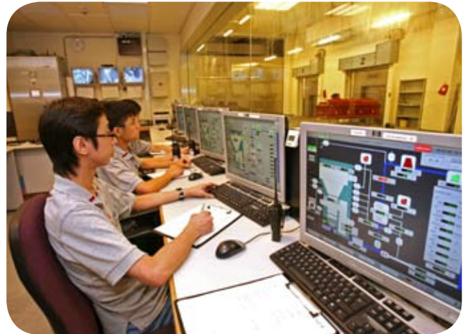
Control room monitoring the operation of cremators in Diamond Hill Crematorium
