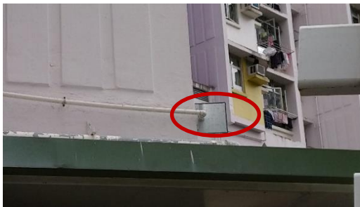
The size of rat guard is too small to screen rodent
