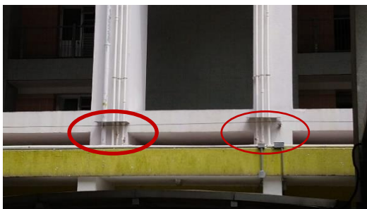
Rat guards installed too near to platform underneath.
